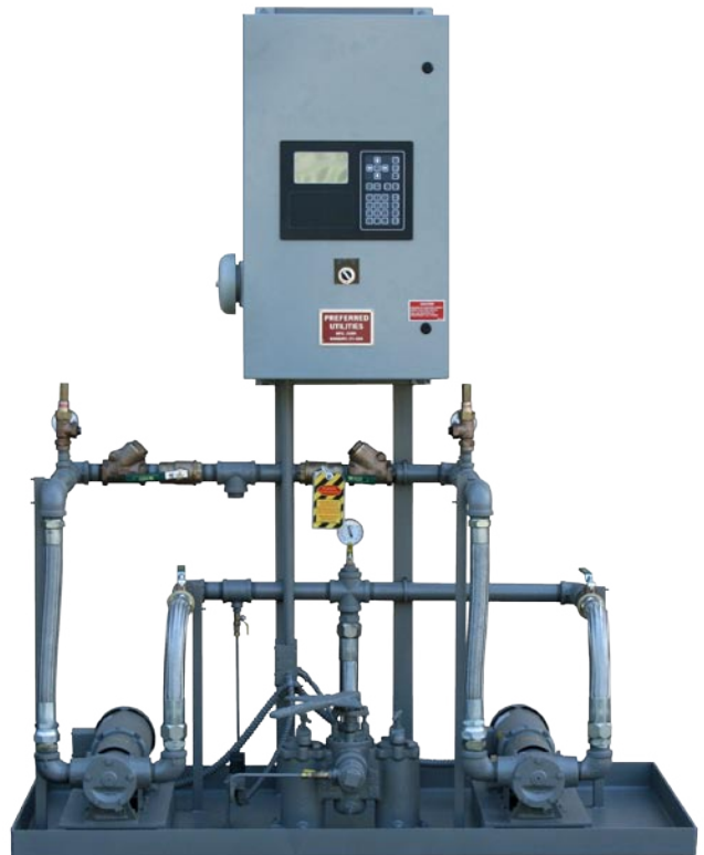
Duplex Pump Set with Inlet Oil Strainer and Pump Control Cabinet
